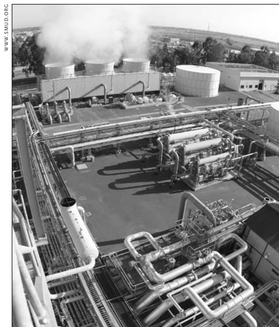
Co-generation “peaker” plants can be used to provide power in times of high demand, such as on hot summer days.
